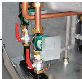
Pumps and gate valves
