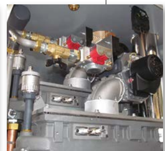
Group of: fan, modulating gas valve, premix burner
